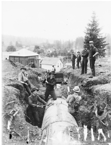
Cedar River Pipeline Number 1 under construction on hill east of Renton, 1899 Courtesy of the Seattle Municipal Archives (Item 7261)
